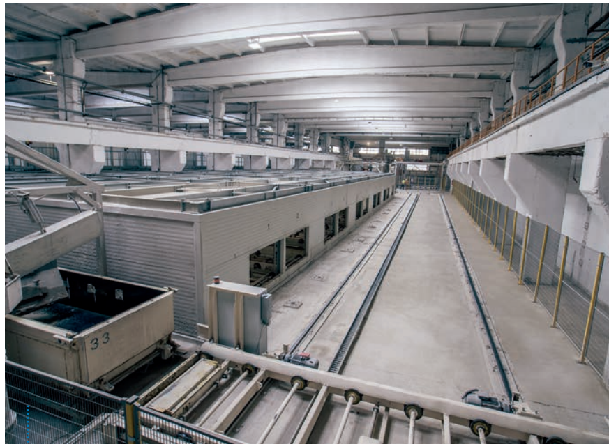
Fig. 2: An overview from the Mixing Tower. Freshly casted moulds are moved fully-automatically to the newly-insulated rising area by the Aircrete traverser car.
