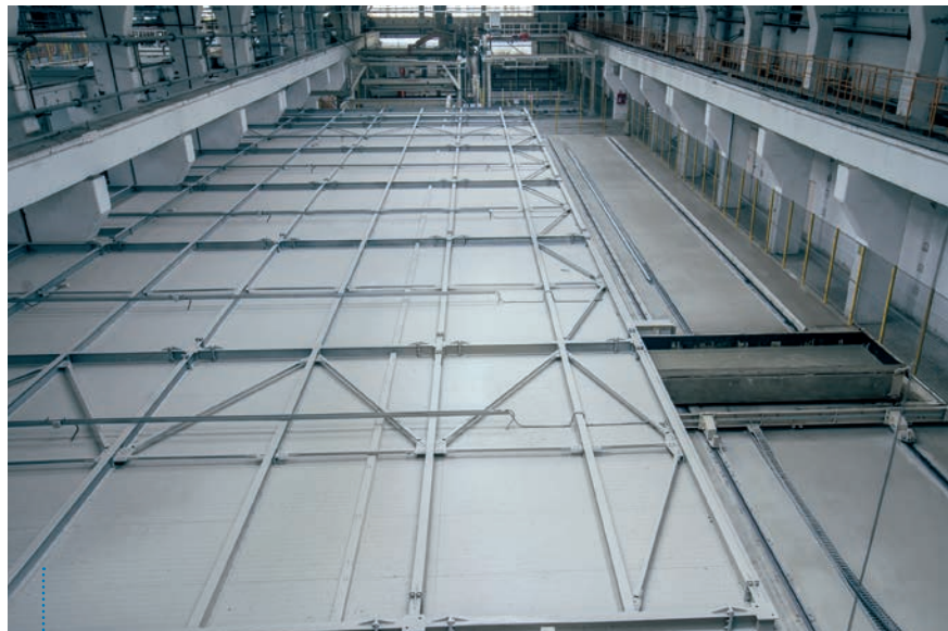
Fig. 3: The new rising area has been covered and fully-equipped with a flexible roller track system.
